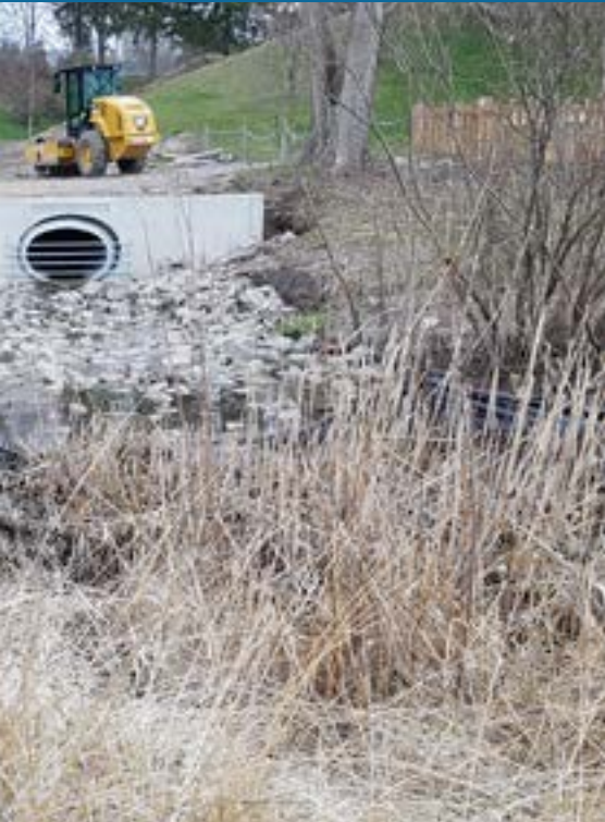
Image of similar project located on the beach in Port Burwell, ON. (Early stages of construction)
